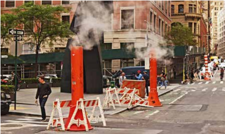
Not very efficient: Steam rises from the underground pipeline system in southern Manhattan.
